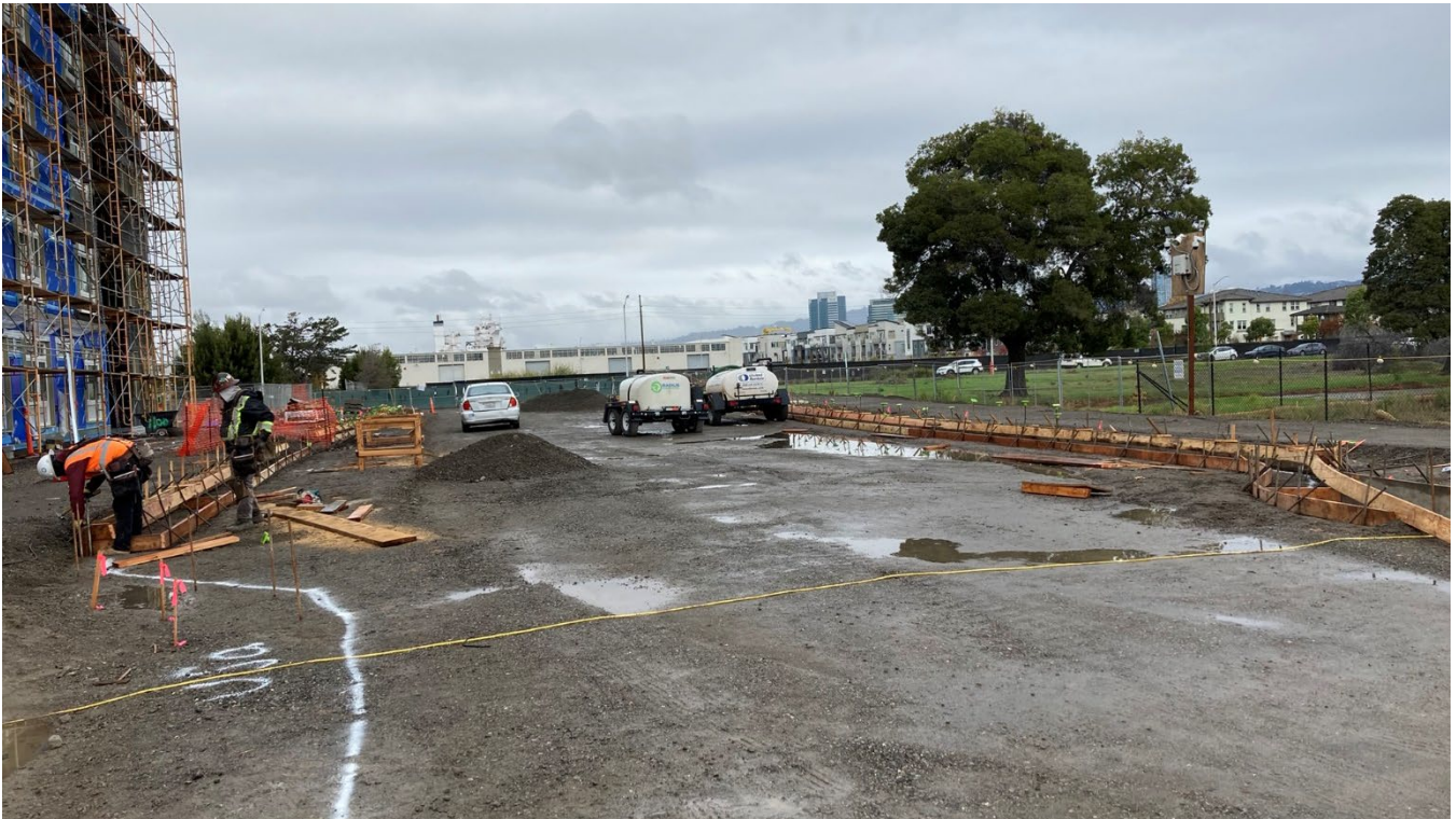
Form work for new curb and gutter at the new Mabuhay Street looking north towards Mosley Ave.
