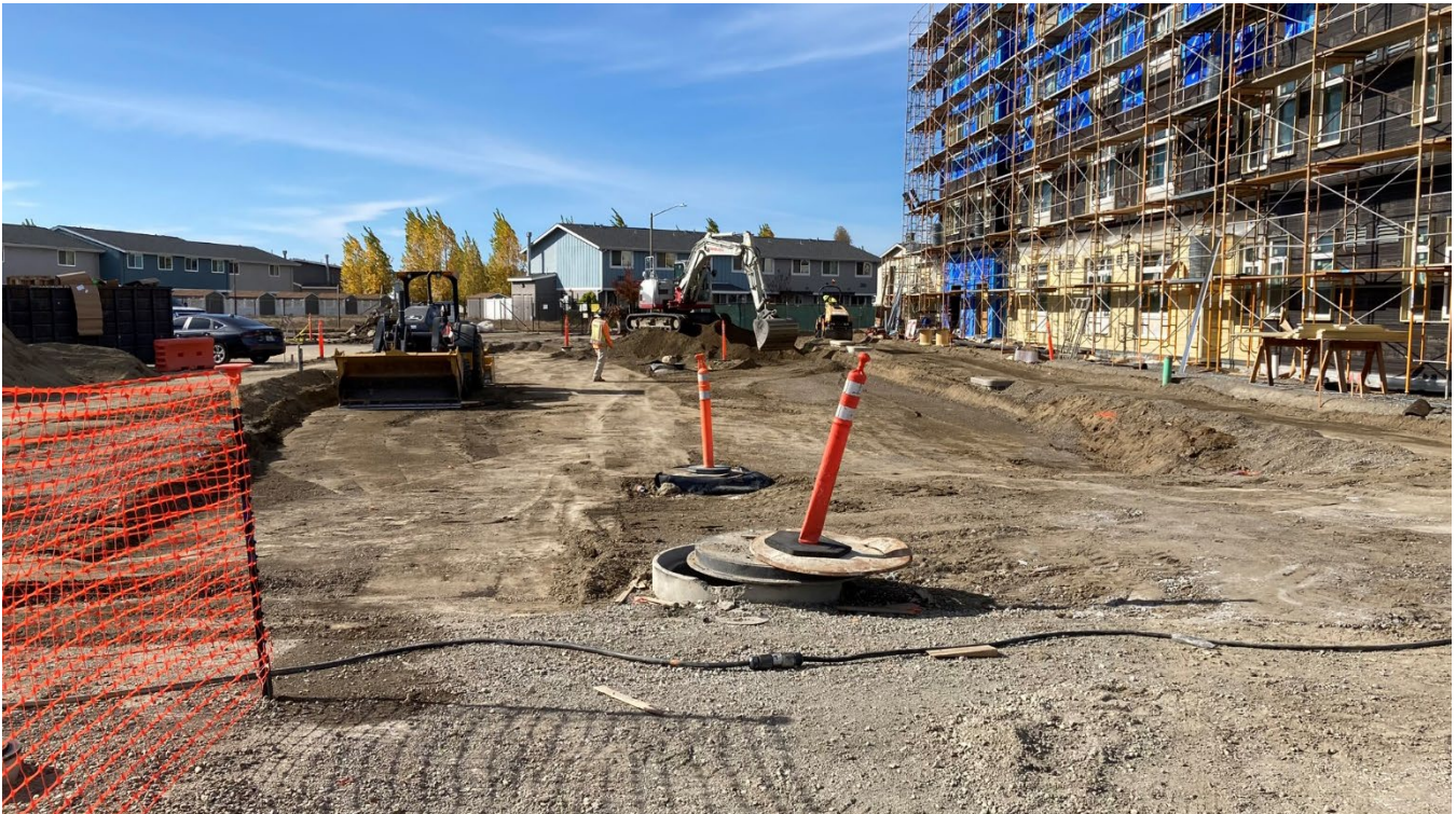
Ongoing grading at the realignment section of Lakehurst Circle, adjacent to Linnet Corner.
