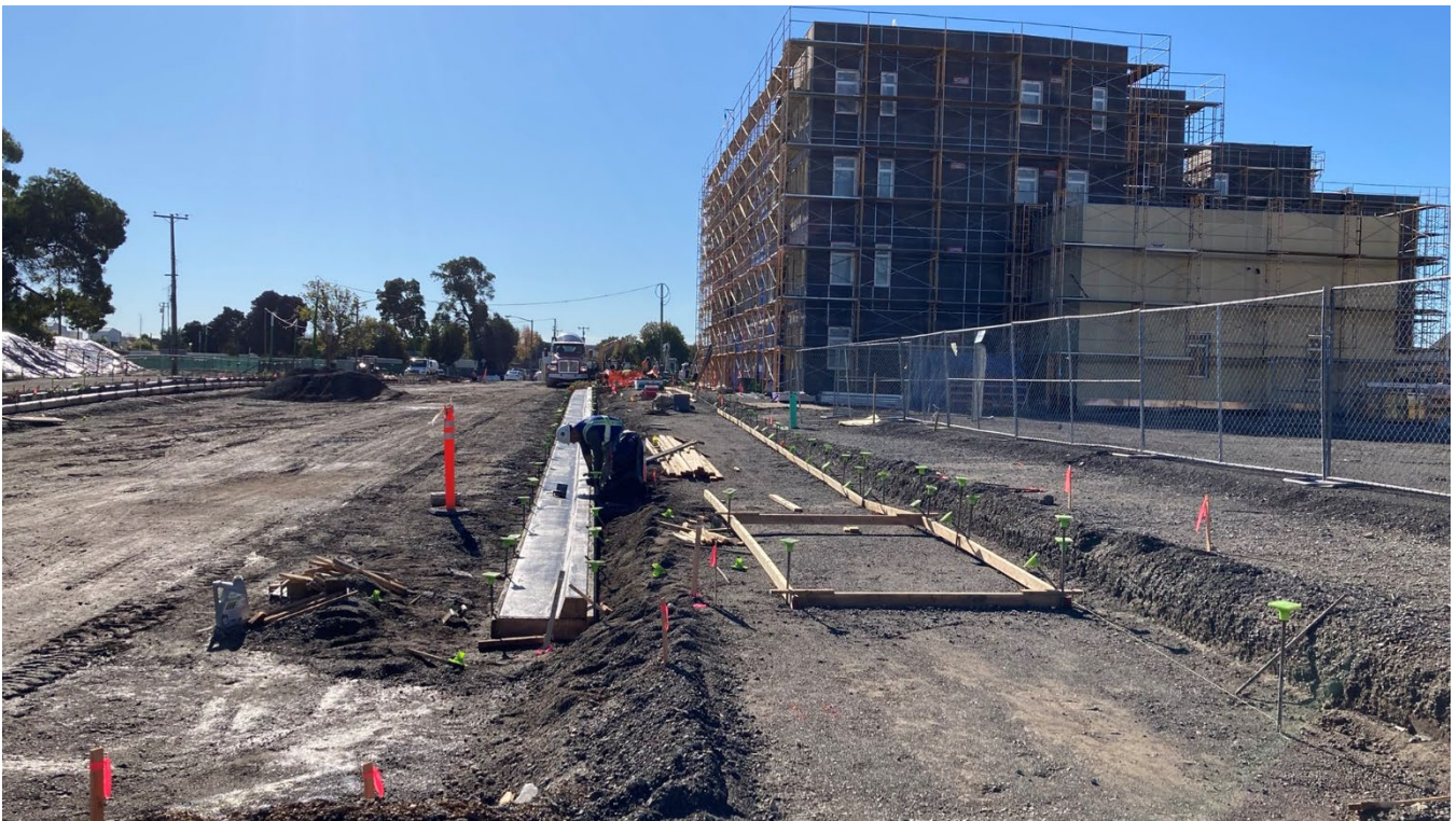
New curb and gutter at the new Mabuhay Street looking south from Mosley Ave, along Estuary II site and Linnet Corner on the right of the photo.
