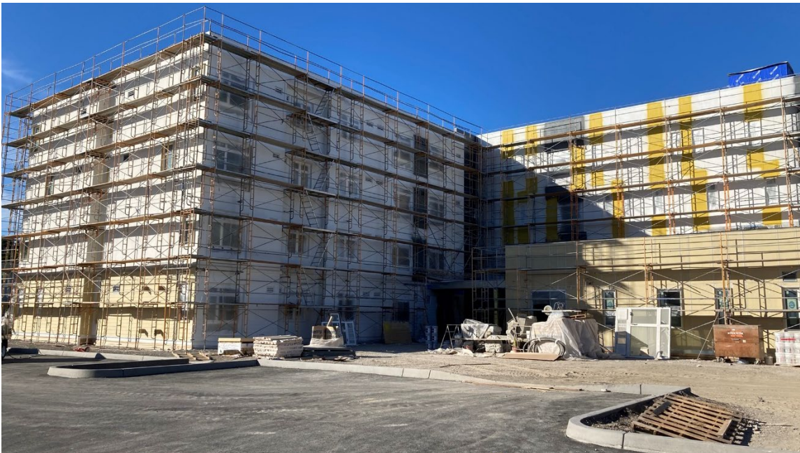
Building progress photo from the southeastern elevation (view from the future parking lot).
